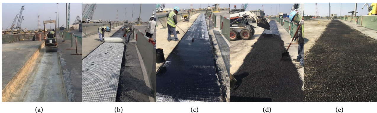
Figure 12. (a) Trench -Compaction of the sub grade, (b) & (c) Laying of Fiberglass grid and application of primer, (d) & (e) Laying of AC layer and compacted pavement.
