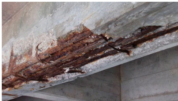
Photo 1. Reinforced concrete beam corrosion [16].
