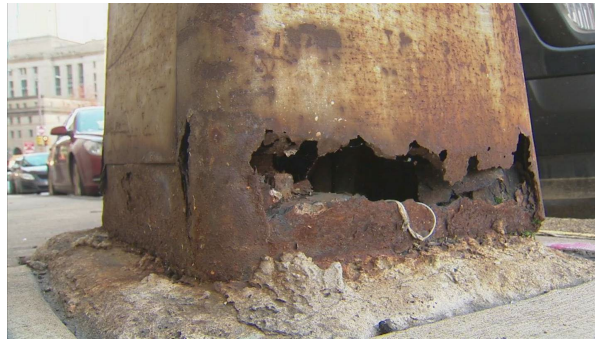
Photo 2. Traffic light corrosion [17].
