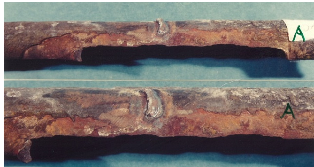
Figure 4. Failed opening exhibited a rectangular slice of the tube material that was lost. A window fracture appearance.
