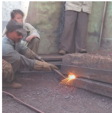
Figure 6. Cutting work being done without protective equipment.
