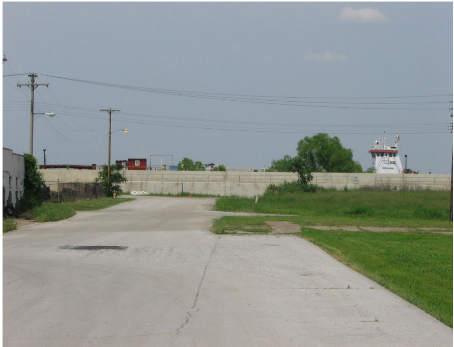
Figure 20. The Cairo floodwall is built on the Ohio River side at the bend in the river where an earthen levee would be difficult to maintain. With the river 3 m above flood stage, a tugboat is visible behind the floodwall. Reprinted with permission from Editor of Journal of Soil and Water Conservation.
