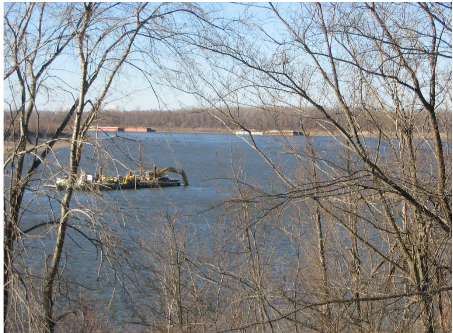
Figure 14. River bottom bedrock is dredged using an excavator to increase the navigation depth. Reprinted with permission from the Editor of the Journal of Soil and Water Conservation.
