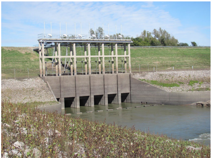
Figure 33. When open, the New Madrid Floodway setback levee gate drains the 80,937-hectare St. Johns Bayou basin to Main Ditch and into the Mississippi River. It is closed under flood conditions to prevent Mississippi River backup water from flowing into the basin. Reprinted with permission from Editor of Journal of Soil and Water Conservation.
