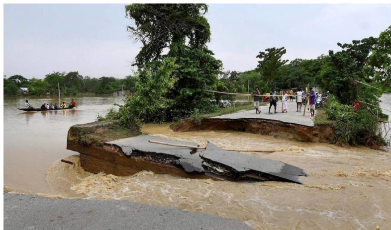
Figure 6. A road in Bangladesh cut by flood water. Photo Credit: Public domain.
