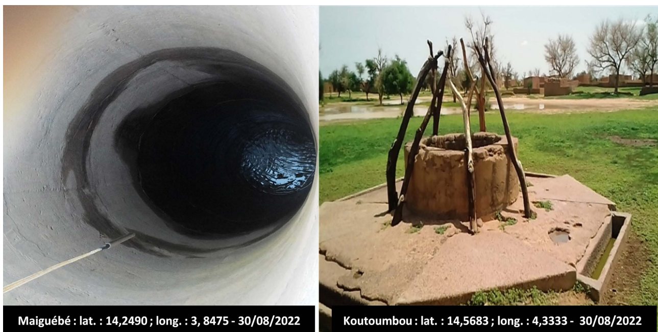
Figure 8. Flooding by lateral intrusion.
