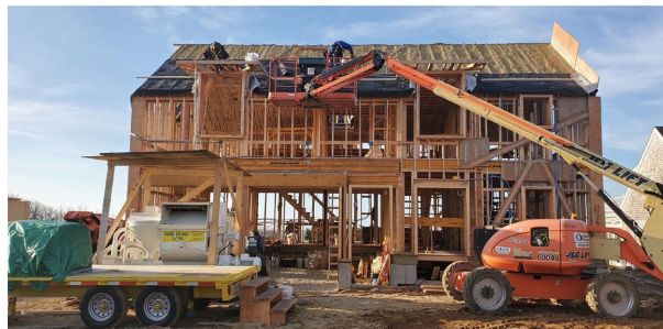
Figure 11. Wood frame of structure before Hempcrete is applied ( https://hempstone.net ; used with permission).
