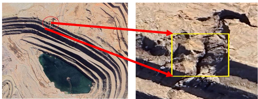
Figure 2. Slope failure image in Mashamba West Mine.
