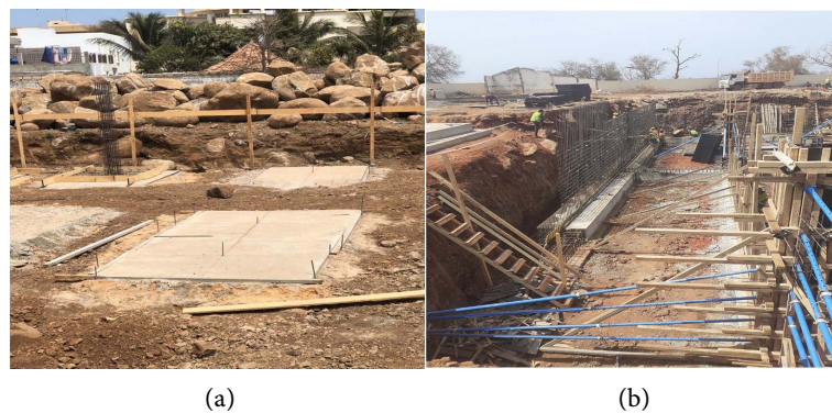
Figure 1. Spread foundations on rock mass ((a) Site Ouakam, (b) Site Almadies, Dakar, Senegal).
