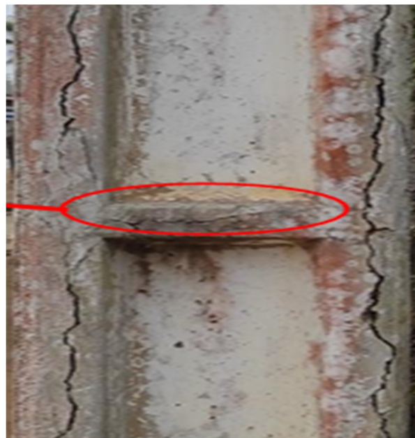
Figure 13. Vertical and horizontal cracks.
