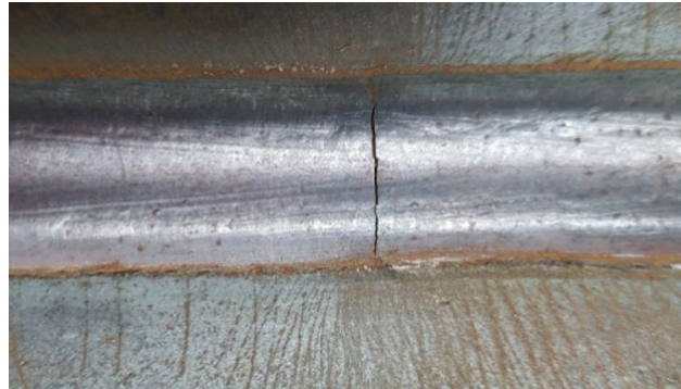
Figure 1. Illustration of a cracked pipeline section retrieved from a field failure.
