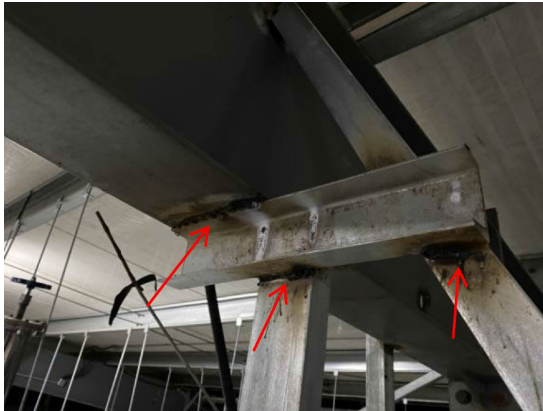
Figure 4. Poor welding quality between the suspended load fixture and the rigid frame.
