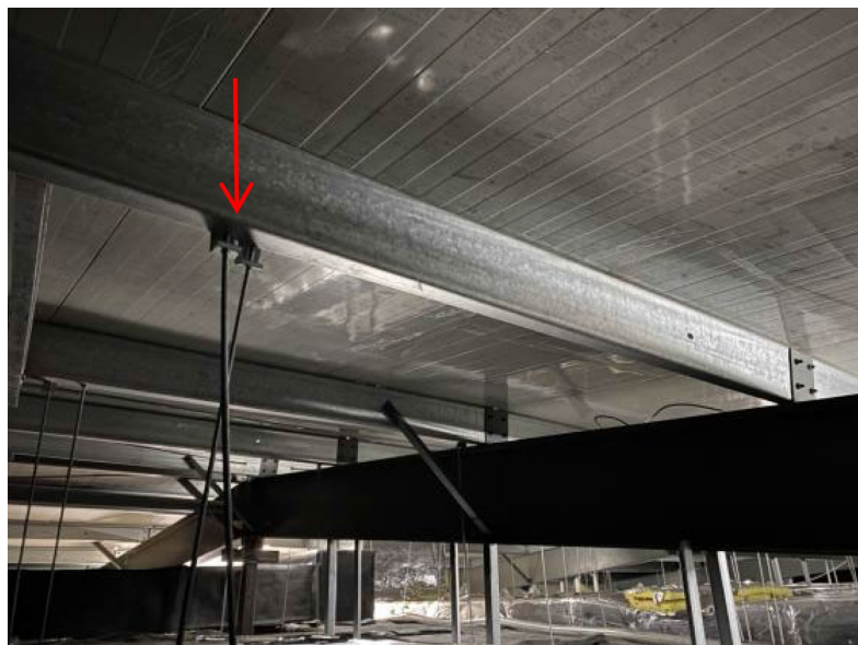
Figure 2. Local considerable deformation of the lower flange of the purlin.
