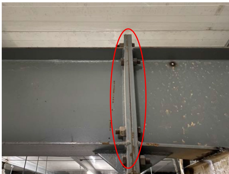
Figure 5. Corrosion of the node bolts of the rigid frame components.
