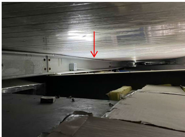
Figure 3. Significant deflection of the purlin.
