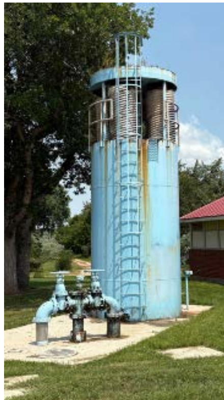
Figure 2. Aeration/degassing tower at McNenny State Fish Hatchery.
