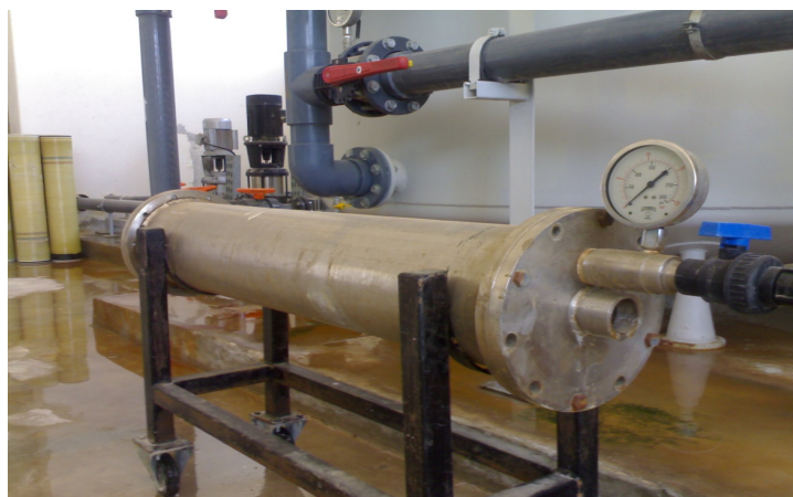
Figure 1. Experimental pilot plant RO unit.
