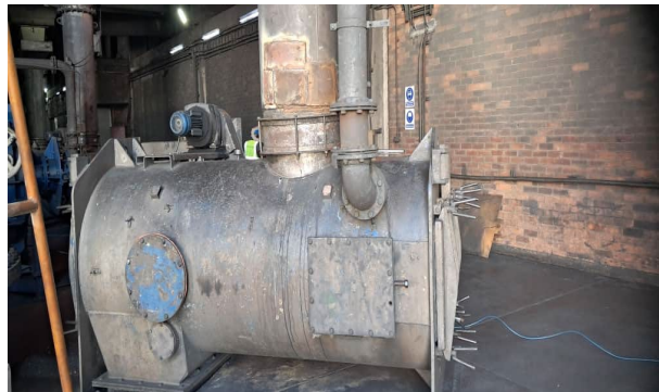
Figure 1. Coal Feeder system.
