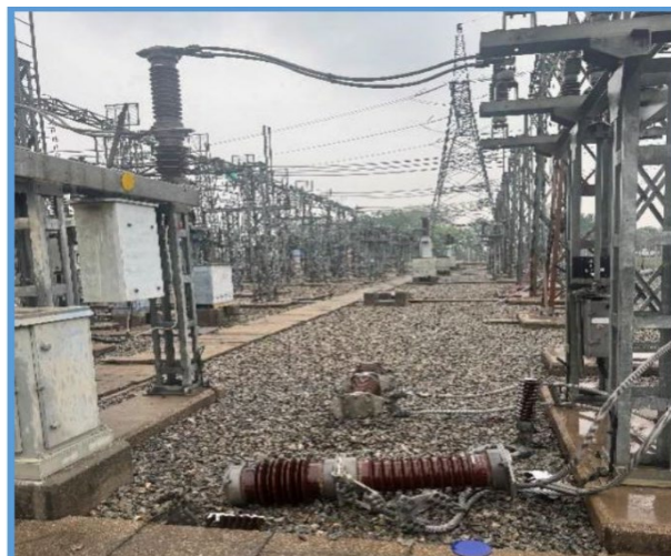
Figure 2. 33 kV Fault breaker fell off after fault.
