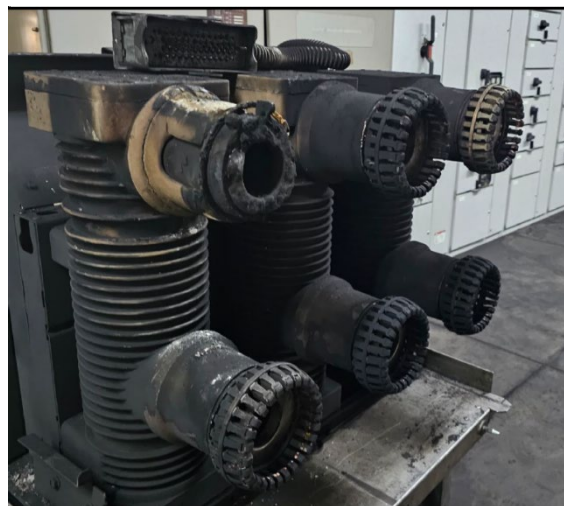
Figure 3. Damaged 3.3Kv Breaker.
