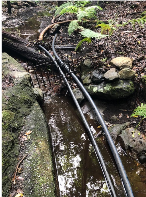
Figure 5. Drainage of Meriga (La Gomera) stream water by means of open canal and pipes (V. Lüderitz).
