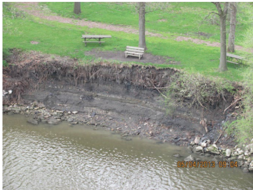
Figure 8. Stream bank erosion at the Illini State Park [2].
