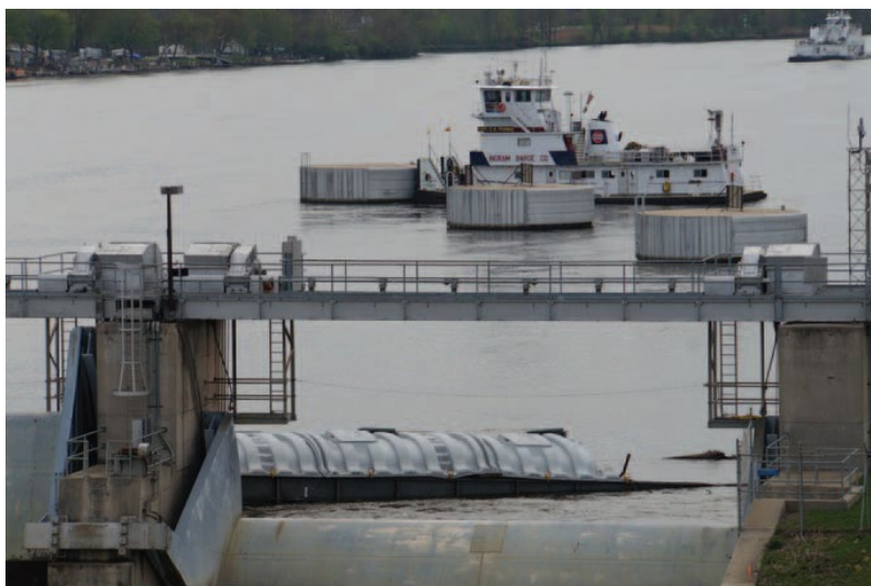
Figure 9. Partially sunken barge and damaged Tainter gates struck at different heights [2].
