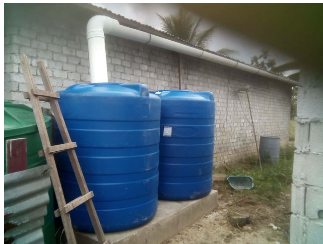
Figure 2. RWHS designed by the team from Swinburne Sarawak in 2019.
