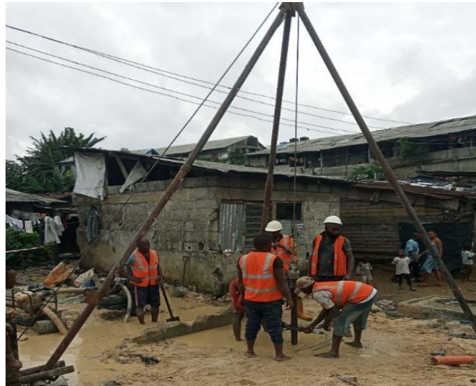
Figure 4. Jetting (Washboring) borehole drilling in one of the project locations (Port Harcourt).
