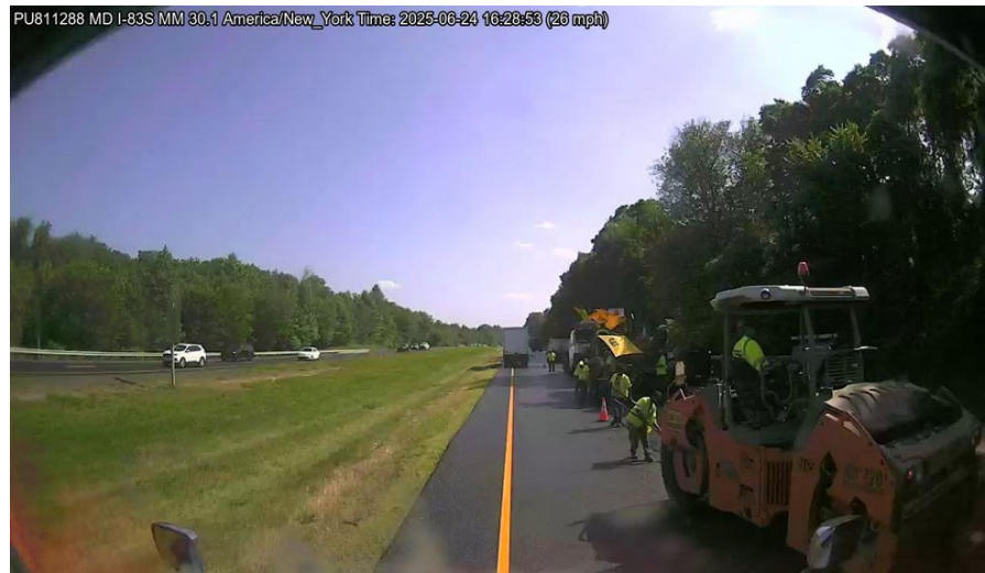
Figure 8. Dash camera image along I-83 in Maryland showing shoulder running due to lane incursions from work crew.
