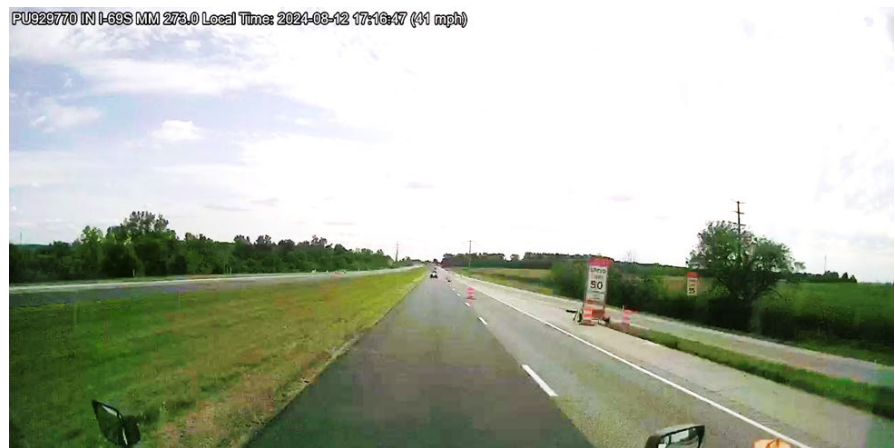
Figure 5. Dash camera image along I-69 in Indiana showing a static work zone speed limit sign and a dynamic work zone speed limit trailer displaying different speed limits.
