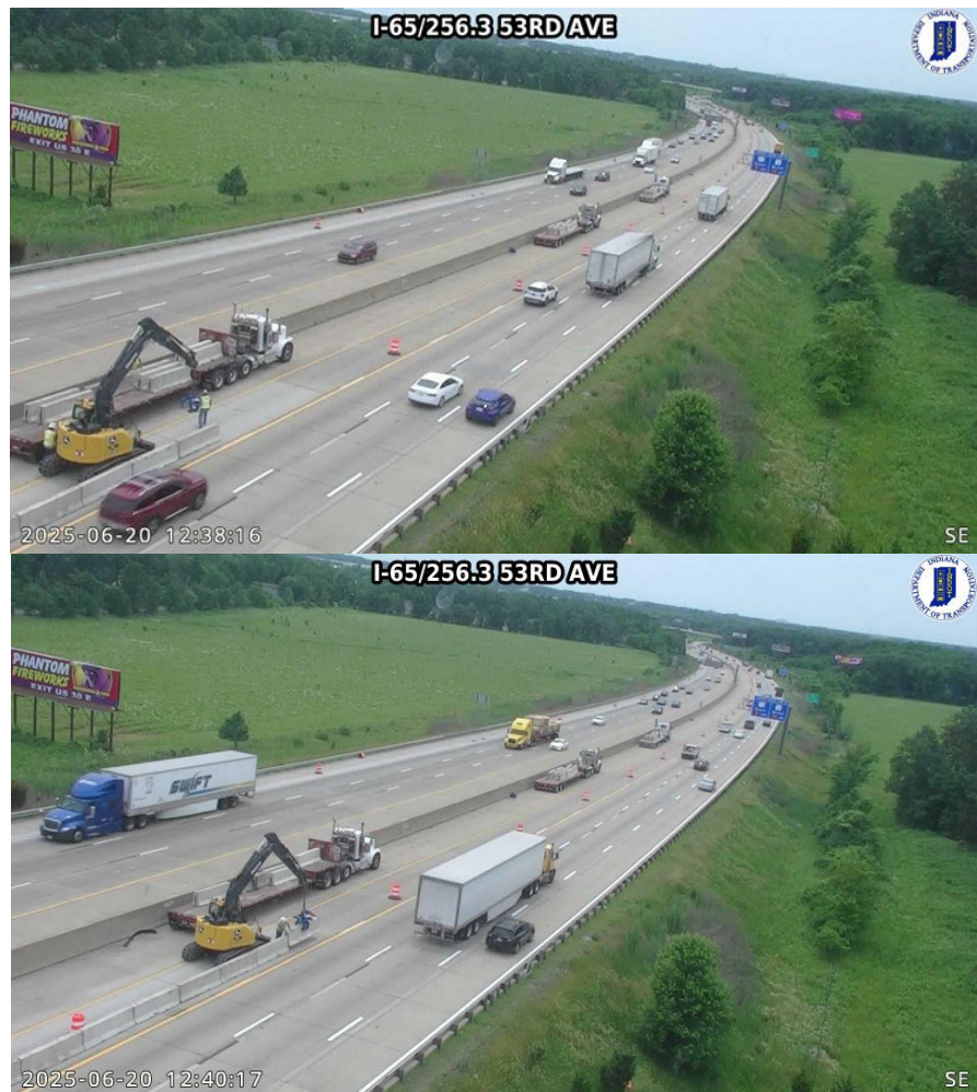
Figure 2. ITS camera images on I-65 in Indiana showing the installation of a concrete barrier wall during the day next to live traffic.
