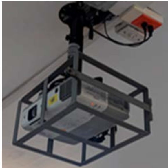
Image 7. Projector mounted on ceiling.
