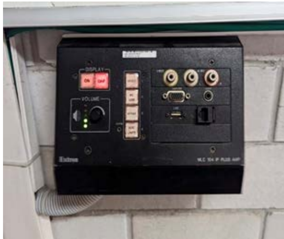
Image 6. Control panel for projector and retractable screen.
