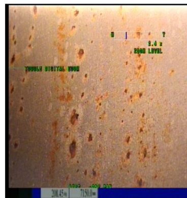
Figure 8. Corrosion and erosion foci concentrated in the zone of bulging by the reinforcing units of the internal housing devices.
