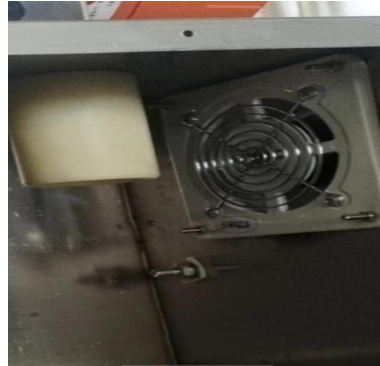
Figure 15. Fan inside picture.
