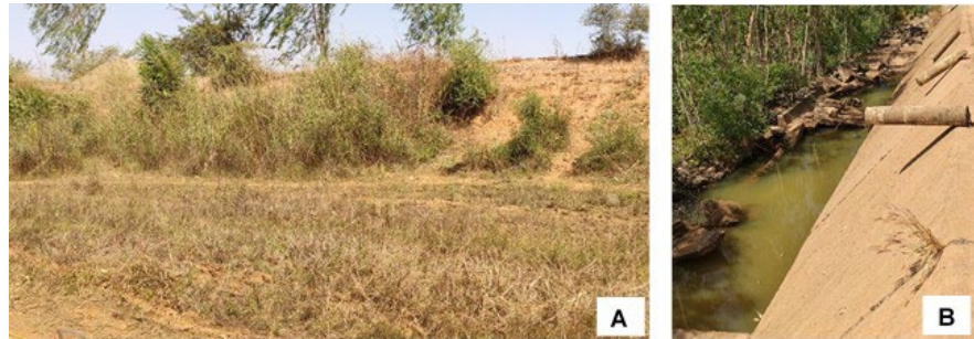
Figure 11. View of areas affected by water leakage. (A) Downstream of the southern section of the embankment. This area remains wet all year round, benefiting the grass and shrubs that persist on the soil and embankment throughout the year. (B) Downstream of the spillway. The persistence of water at this location during the dry season (February) indicates the presence of water leaks below the spillway. The damage we also observe there, is doubtless partly caused by these leaks.
