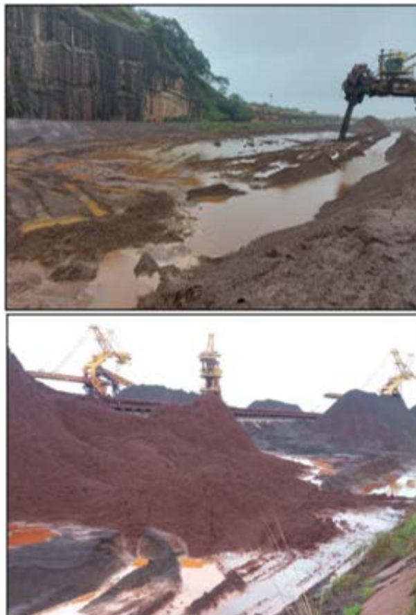
Figure 6. Stockyard foundation with low bearing capacity.
