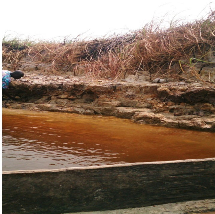
Figure 11. Erosion following desiccation of clayey soil.
