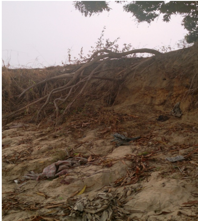
Figure 8. Sliding and scouring on silty soil.
