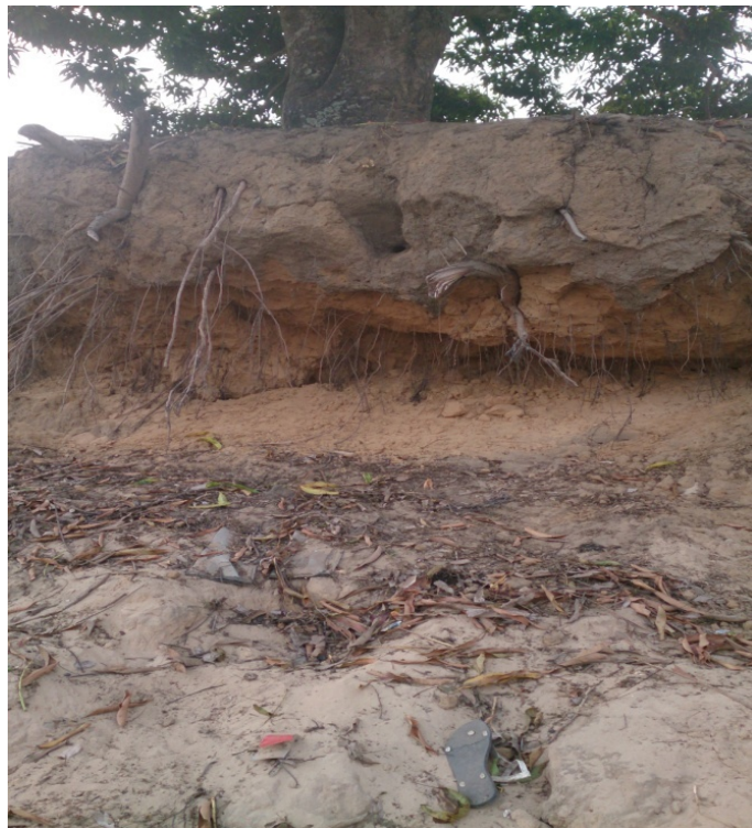
Figure 9. Scouring sequence of riverbanks causing landslides of silty soils.
