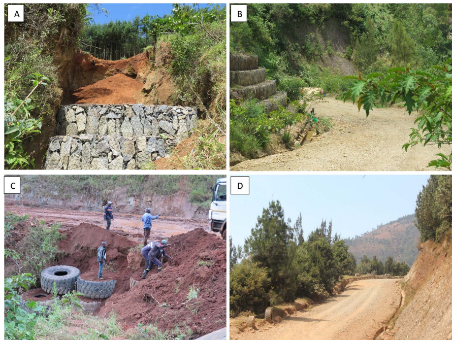
Figure 2. Gabion baskets in support of the main access road (A) and a wall side (B); tires being positioned to support an access road with drainage (C) and concrete side drains on the wall side (D).
