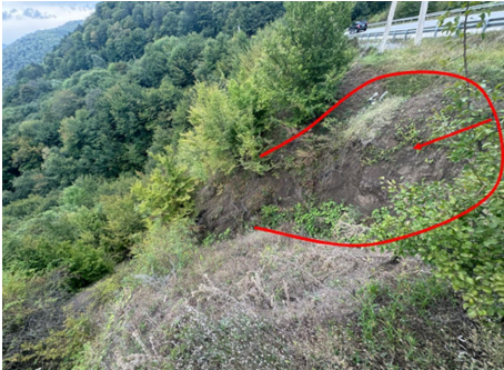
Figure 6. Main rupture of the landslide (#4).
