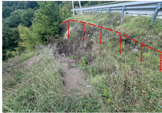
Figure 8. The main rupture stage of the landslide body, which is close to the roadway.
