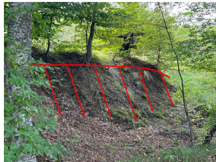
Figure 11. Fragment of the main landslide cutoff.
