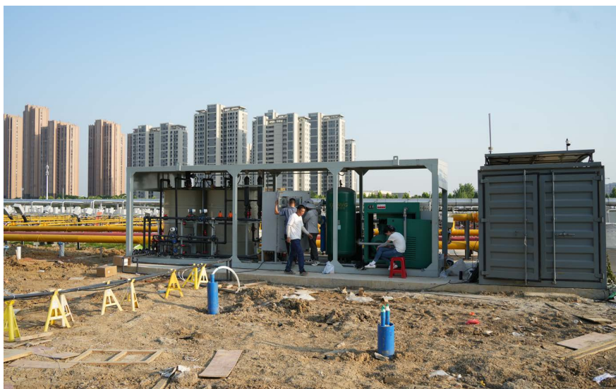
Figure 8. GCW processing site located in Hefei, China.
