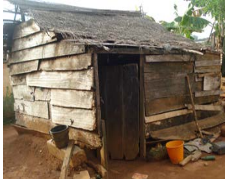
Figure 8. Deteriorated wooden structure.
