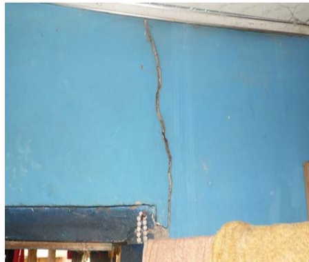
Figure 6. Vertical crack from lintel to door frame.
