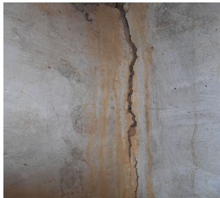
Figure 5. Vertical through crack on cement rendered landcrete wall.
