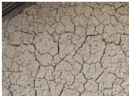
Figure 3. Crocodile skin cracks on landcrete wall.
