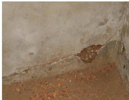
Figure 4. Spalling-off on cement rendered landcrete wall.
