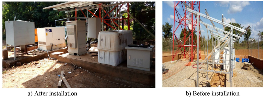
Photo 1. General view of the Gounghin ZI telecommunications site.
