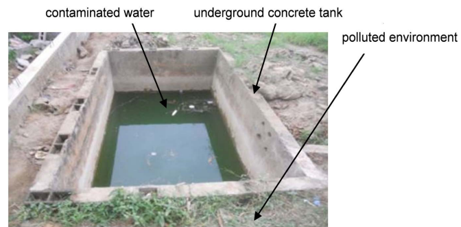
Figure 1. Concrete wall and sealing problem, infiltration of groundwater into the reservoir [13].
