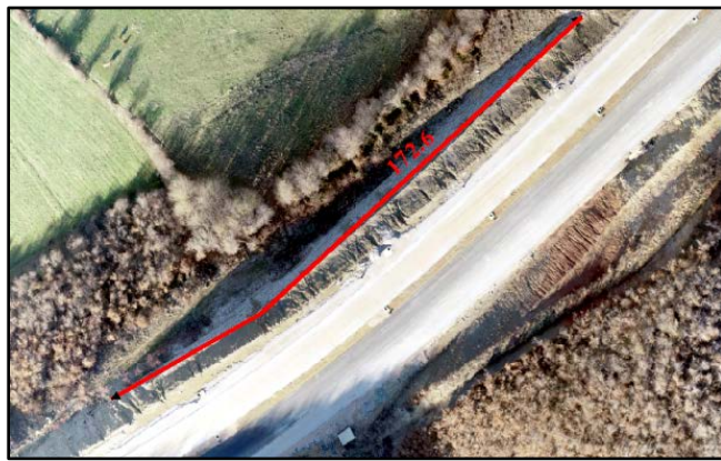
Figure 8. Designed gabion wall and Top view of gabion retaining wall, its actual length.
