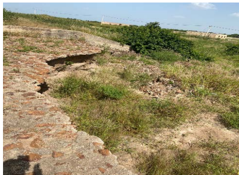
Figure 10. Rupture at the down stream slop.
