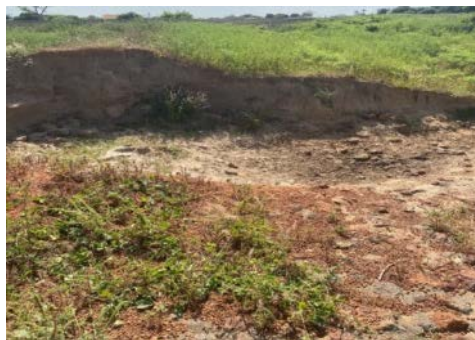
Figure 11. Rupture at the spillway.
