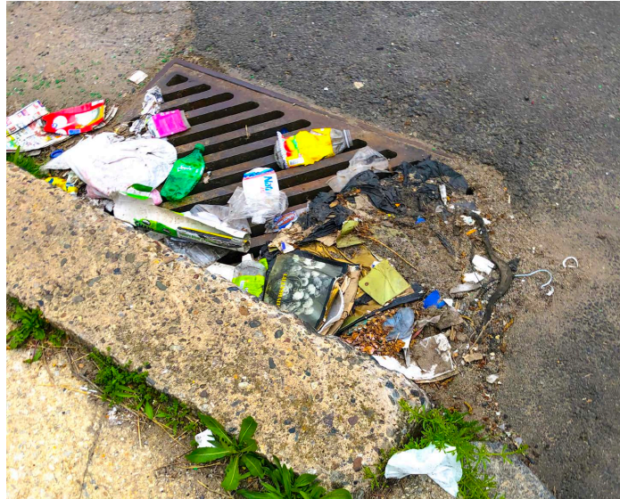
Figure 2. Litter items trapped by a drain grate (Philadelphia).
