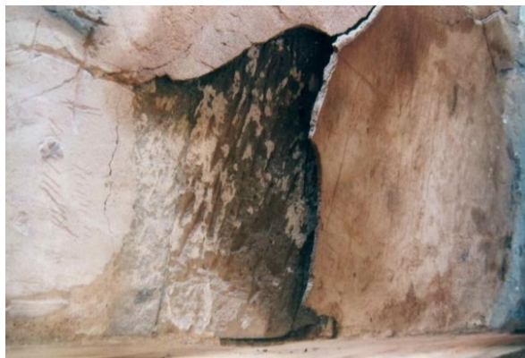
Figure 8. Plaster that splits and cracks from the wall (Bengül, 2005).
