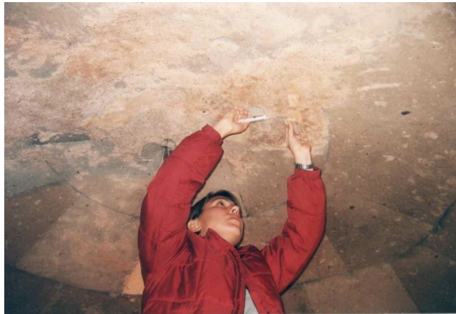
Figure 10. Consolidation of the plaster by injecting primal SF 016 with the help of an injector (Bengül, 2005).
