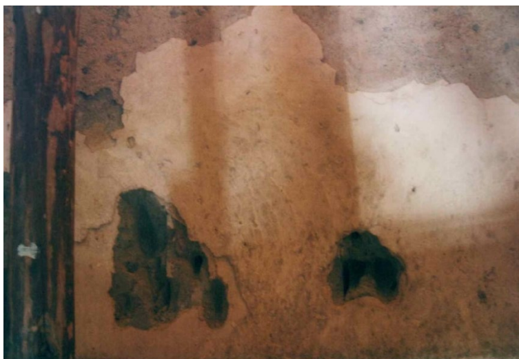
Figure 19. Holes made by bullet holes in plaster and walls (Bengül, 2005).
