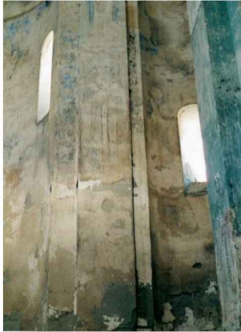
Figure 5. Deteriorations of plasters (Bengül, 2005).
