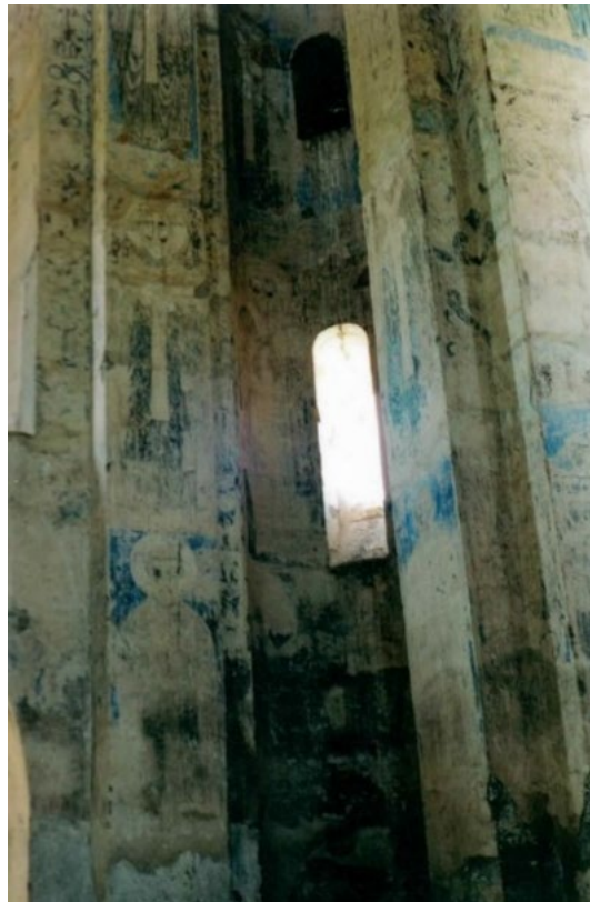
Figure 4. The church walls before repairing (Bengül, 2005).
