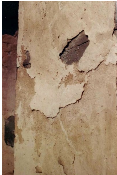
Figure 7. Swelling and flaking plasters (Bengül, 2005).
