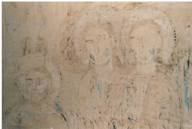
Figure 18. Deterioration of the wall paintings (Bengül, 2005).
