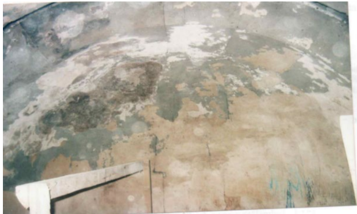
Figure 9. Plaster losses in the dome and rotting of the plaster due to moisture (Bengül, 2005).
