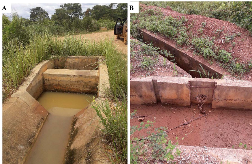
Figure 2. Intake structures for water supply at the level of the irrigated area of M’Bahiakro: (A) Concrete canal; (B) Earth canal.
